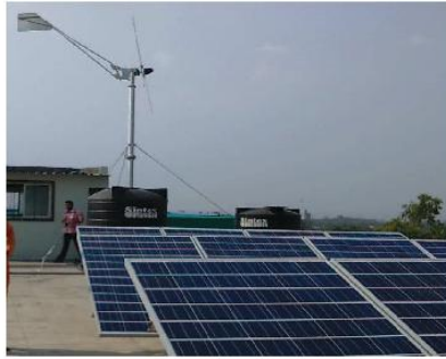
Solar-Wind Hybrid Power Generation Plant
